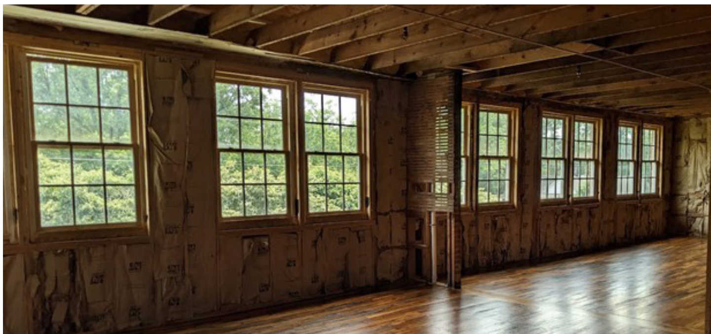
Part of the Winterville Cultural Center (formerly the Winterville High School) currently undergoing renovation and restoration.
